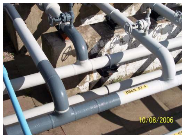
Typical pipe work after painting
